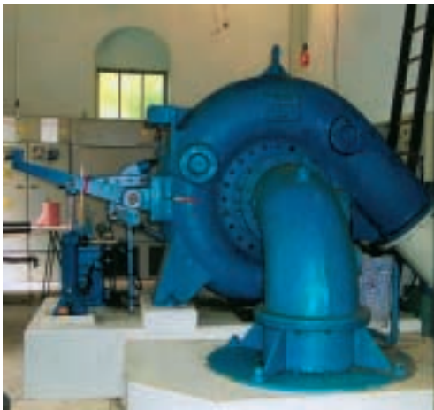
Deux turbines Banki (cross-flow)
